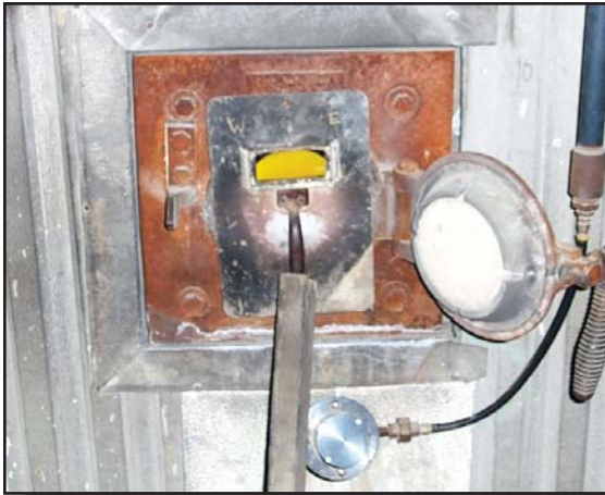
View through access point on the boiler wall. Coal powered boiler temperatures can range from 2200-2500°F, which creates high demands for cleaning equipment.
